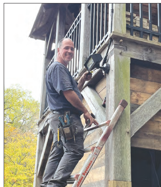
Bill Tinker of Hardwick, master electrician, volunteered to make repairs to electrical wiring and installed floodlights outside and lights inside the gazebo at New Furnace Landing, part of Ware River Park in Gilbertville.
