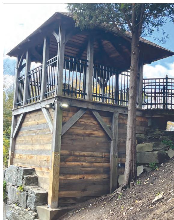
The underside of the gazebo was enclosed to protect it from vandalism and littering.
