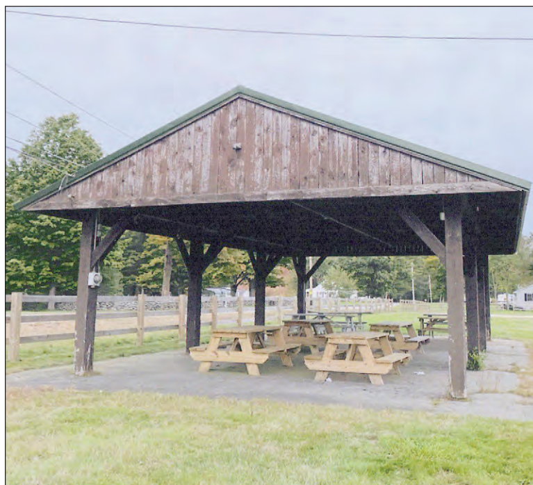
A photo of the pavilion before Hunter Casey began his Eagle project.
