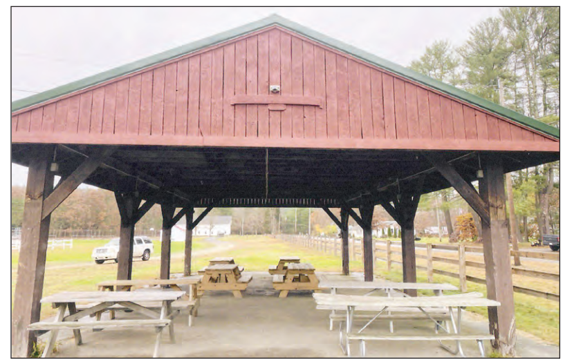
Submitted photos The second part of Hunter Casey's Eagle project was the repairing and painting of the pavilion at Felton Field in Barre.
