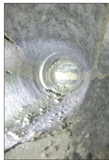
Here is the view while coring into stone (one of 32, three-inch cores to hold new steel reinforcements and bonding grout).
