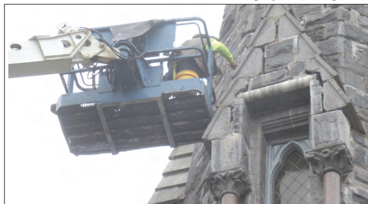
Workers are shown sealing lantern level exterior, which is necessary to keep new grout from seeping out of deteriorated masonry.
